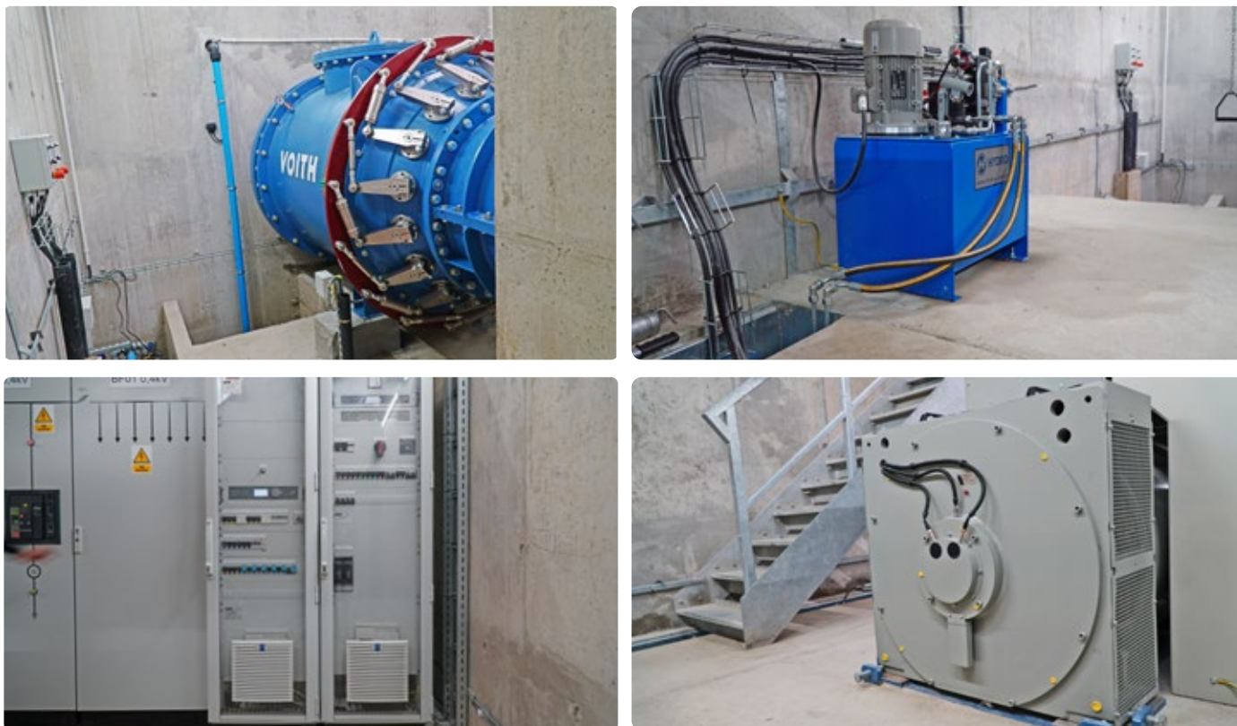
Photo 3. Key elements of the SHP equipment: water turbine, hydraulic power pack, electrical cabinets/turbine automation, synchronous generator
